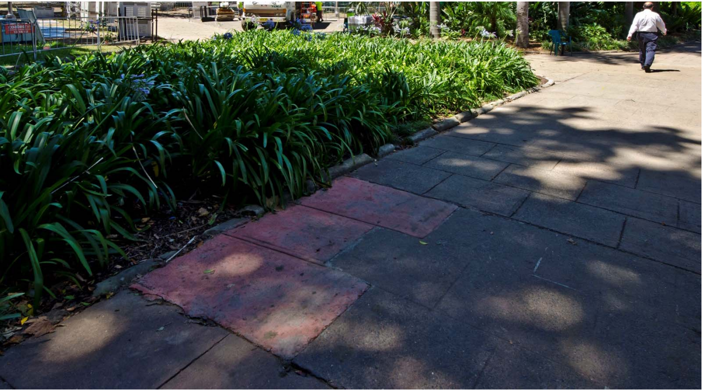
Image e) Broken pavers patched with coloured concrete
