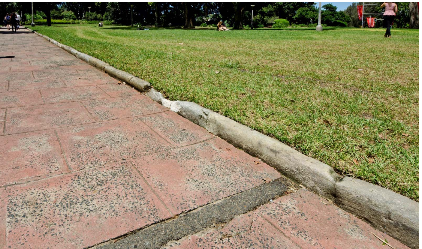
Image d) Broken sandstone edging and asphalt patched pavement
