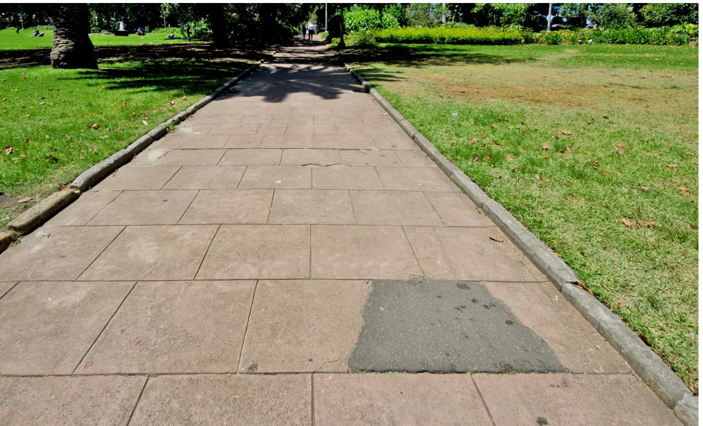
Image f) Broken pavers patched with asphalt
